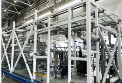
Mechanical oil sludge dewatering unit
