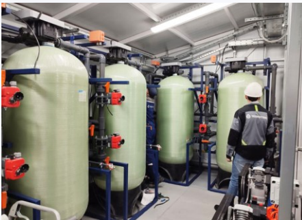
Block-modular water treatment complex
