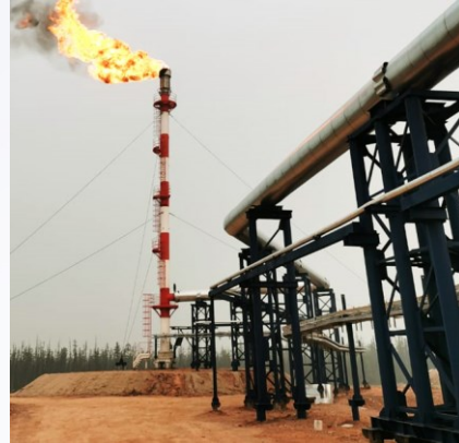
Flare and ignition system
