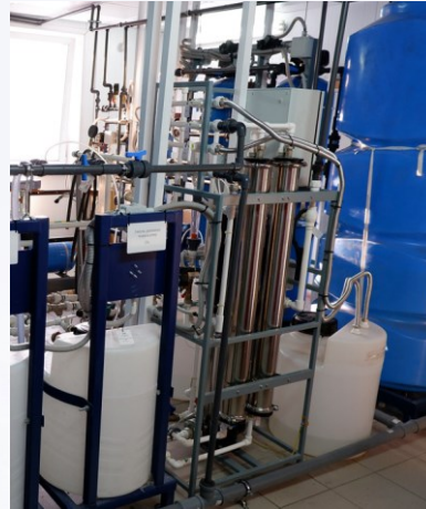
Potable water treatment unit
