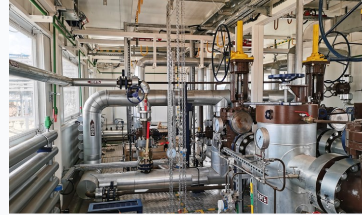
Oil quantity measurement system
