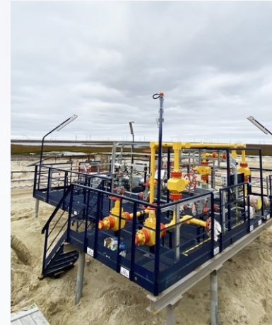
Shut-off valve assemblies
