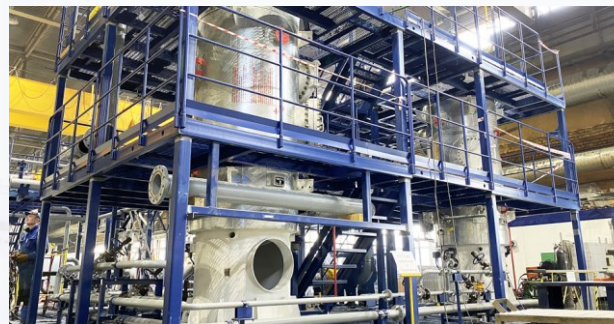
Gas Treatment Unit
